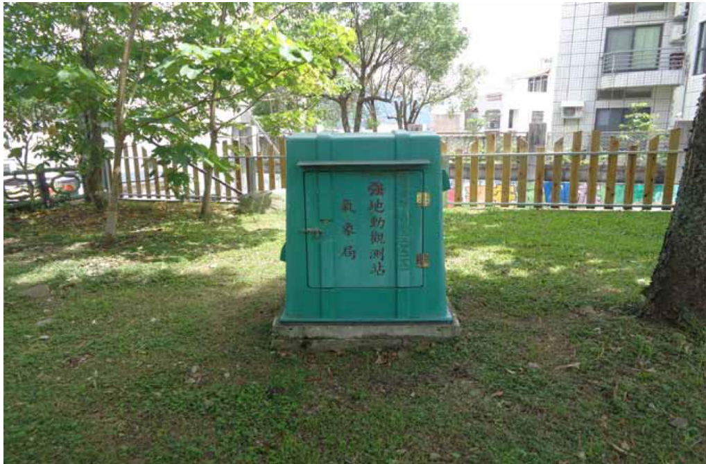
Fig. 17 Station F004 was deployed exactly at the free field on the surface. The picture is from the GDMS database
